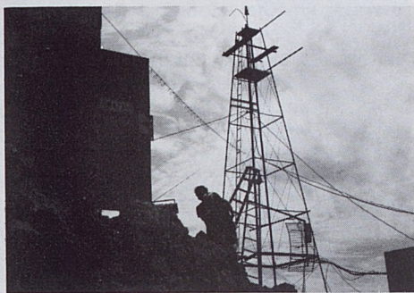
Mike Worrall, KNPR's chief engineer, shoulders the cable which will transmit the station's signal through this new translator, located in Moapa Valley.
