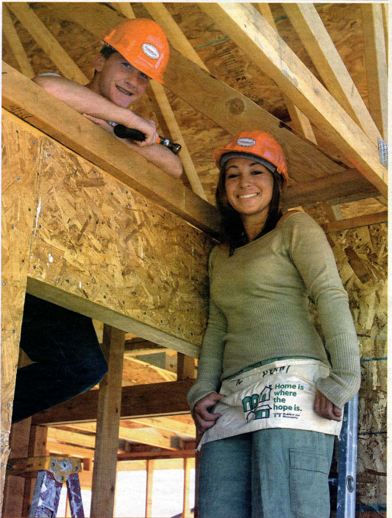
Western High School sophomores Jonathan Sprik and Colleen Montes hang out at one of the houses under construction by Habitat for Humanity.
