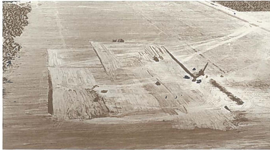
McNeil Construction Company cleared large sections of the desert for the BMI facility, circa 1941
