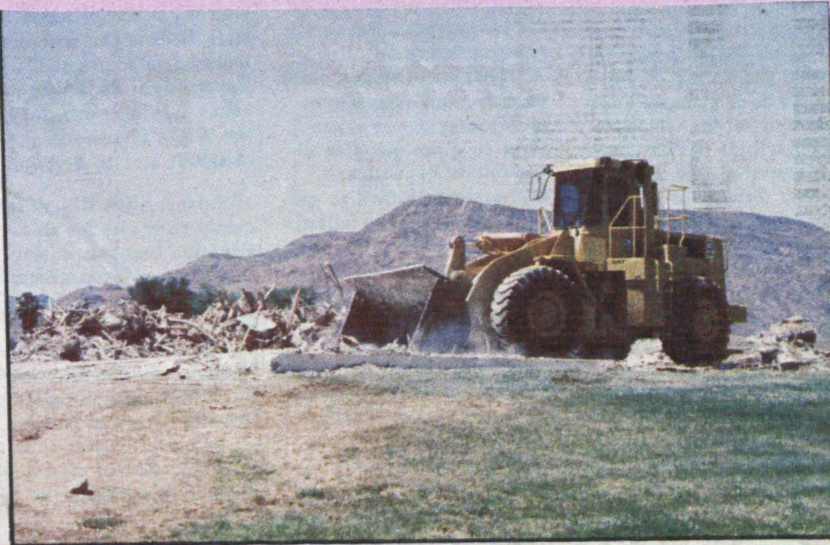
FIRST STEP —Demolition of several buildings at the Civic Center site of the new city hall began last week. Completion of a new city building and library is expected by late summer 1987.
