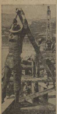
Manpower gets busy as these U. S. army engineers build bridges that connect up with the Alcan highway.
