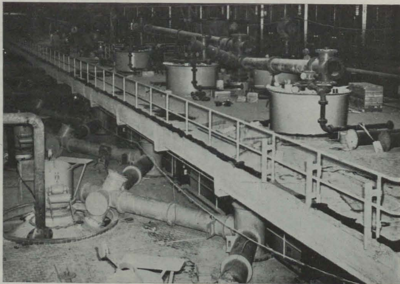
TOPS OF CHLORINATORS, in a row at left, include a charging device for feeding material with minimum escape of gas. At right are exhaust gas scrubbing towers in which magnesium chloride and acid vapors are removed from chlorinator fumes
