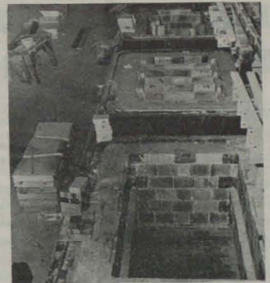
Construction view. Cell tanks are refractory-lined steel arranged in eight rows of eleven
