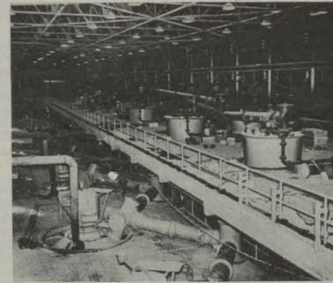
Tops of chlorinators, left, include a charging device which minimizes escape of gas. At right are exhaust gas scrubbing towers
