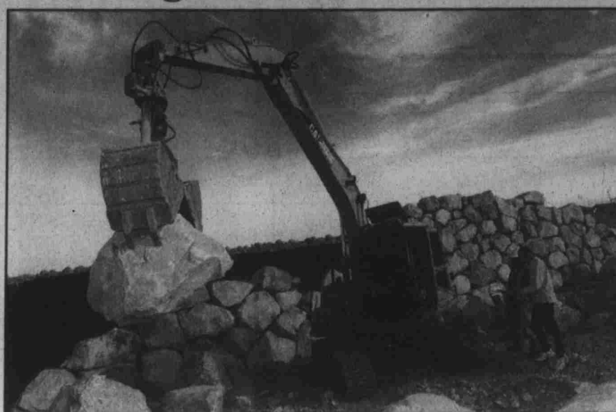
Parsons Bros. Rockeries has moved its headquarters to a new location. Kevin Parsons, right, president of Parsons Bros., talks to Irie Shriver. The operator of the equipment is Ken Johnson.
