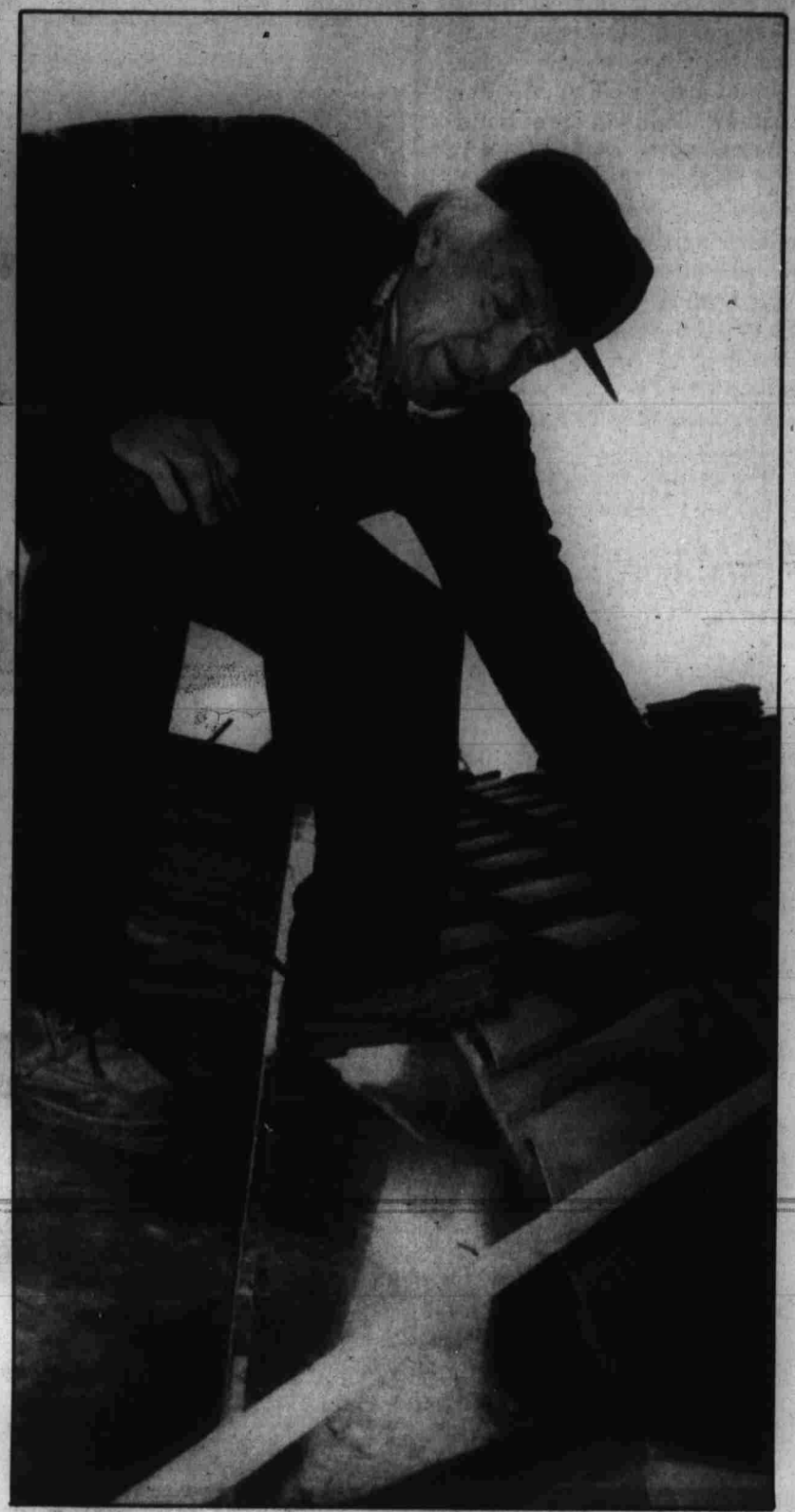
Habitat for Humanity construction coordinator Norm Jacobson keeps his balance while marking roof tiles to be cut.
