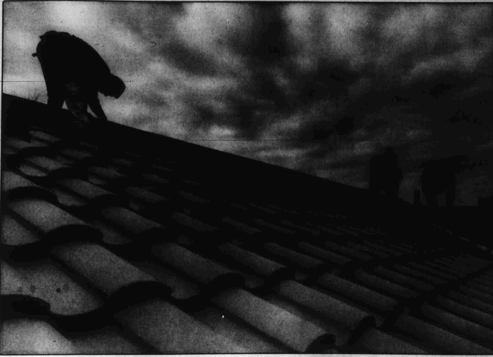
Several Habitat for Humanity volunteers work on the roof of the Ashcraft's new home on Evelyn Avenue.
