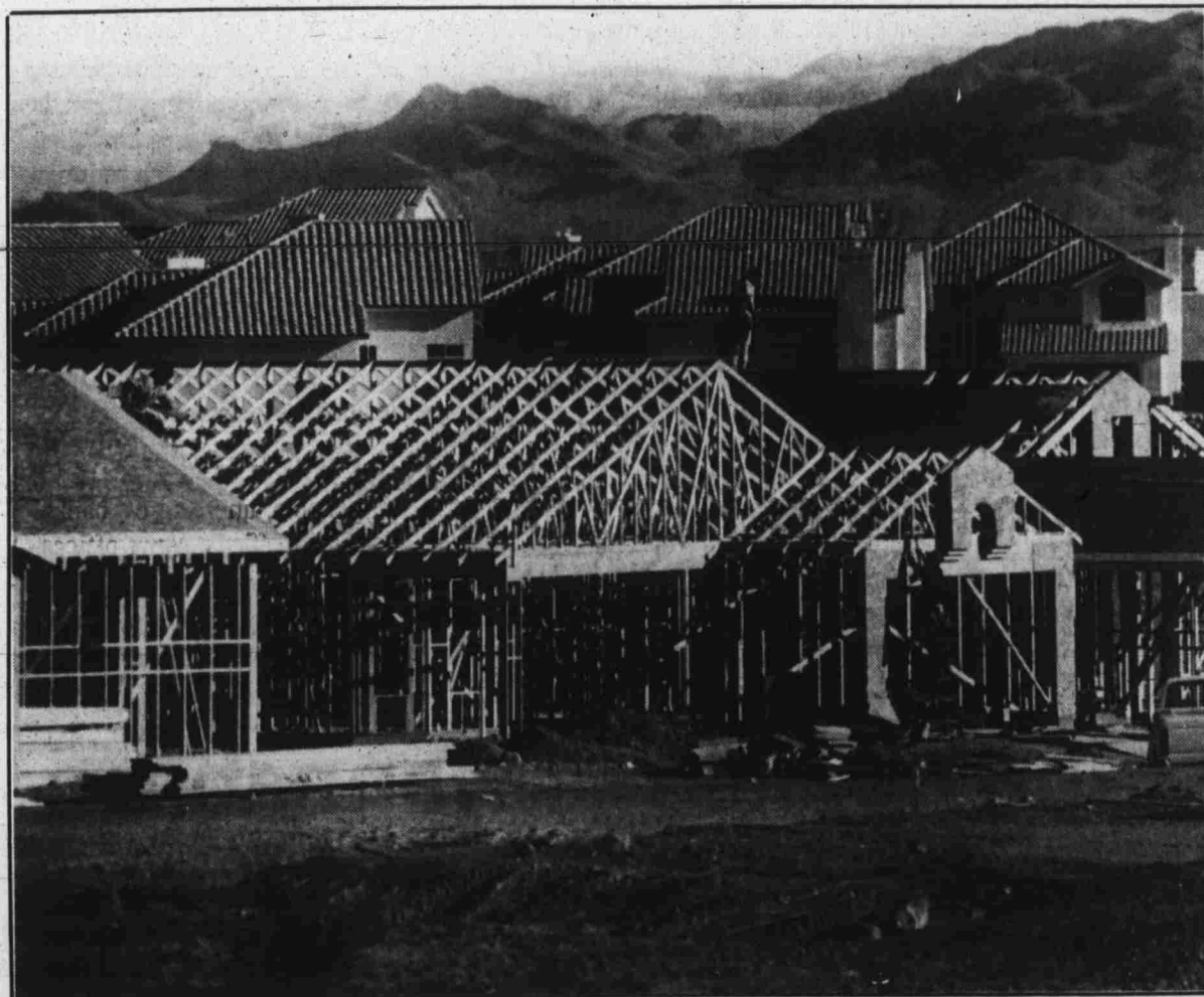
RESIDENTIAL GROWTH — A worker stands atop a framed house in the Green Valley neighborhood's Coral Ridge development. Planning director George Garcia said to expect continued growth in all areas of the city as well as diversified multi-family projects. Photo by Brian Jones
