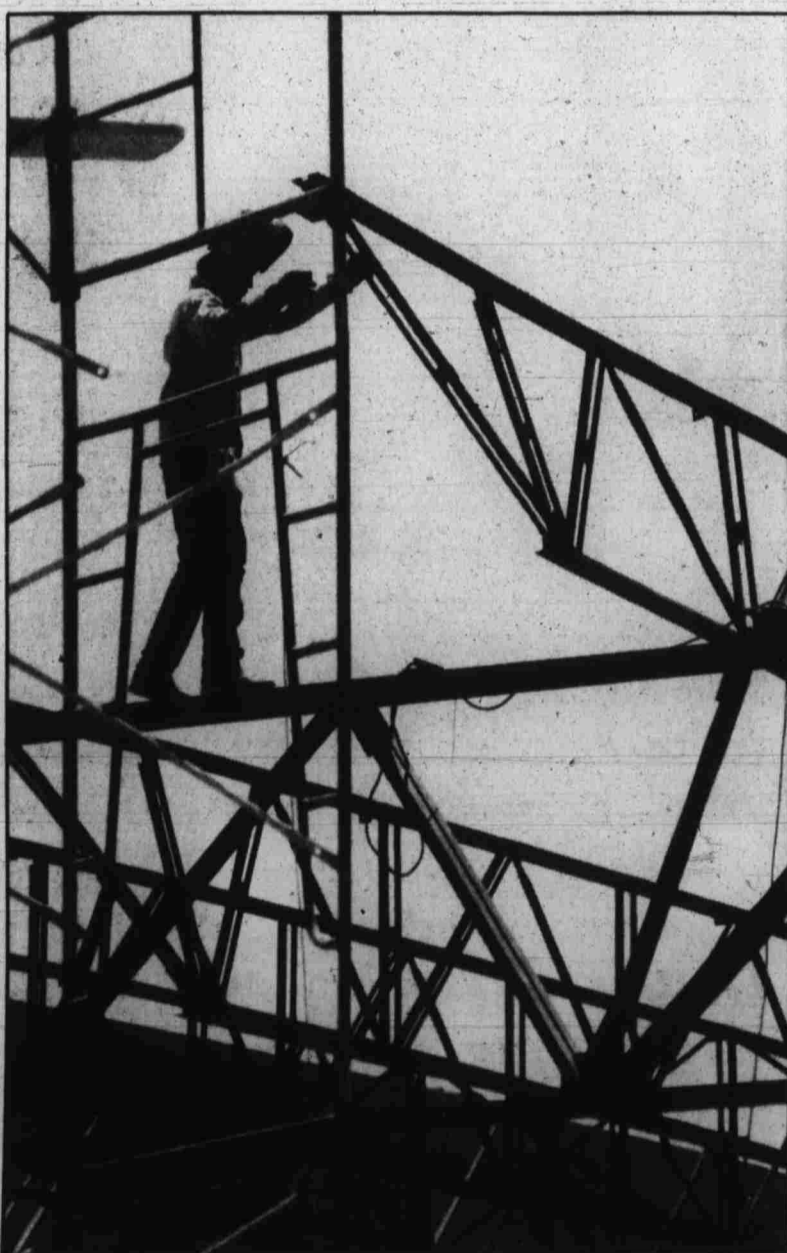
TIGHTWALK — A construction worker balances on scaffolding at the Wal-Mart currently under construction at the Victory Village Plaza. The store will create 245 new jobs.
