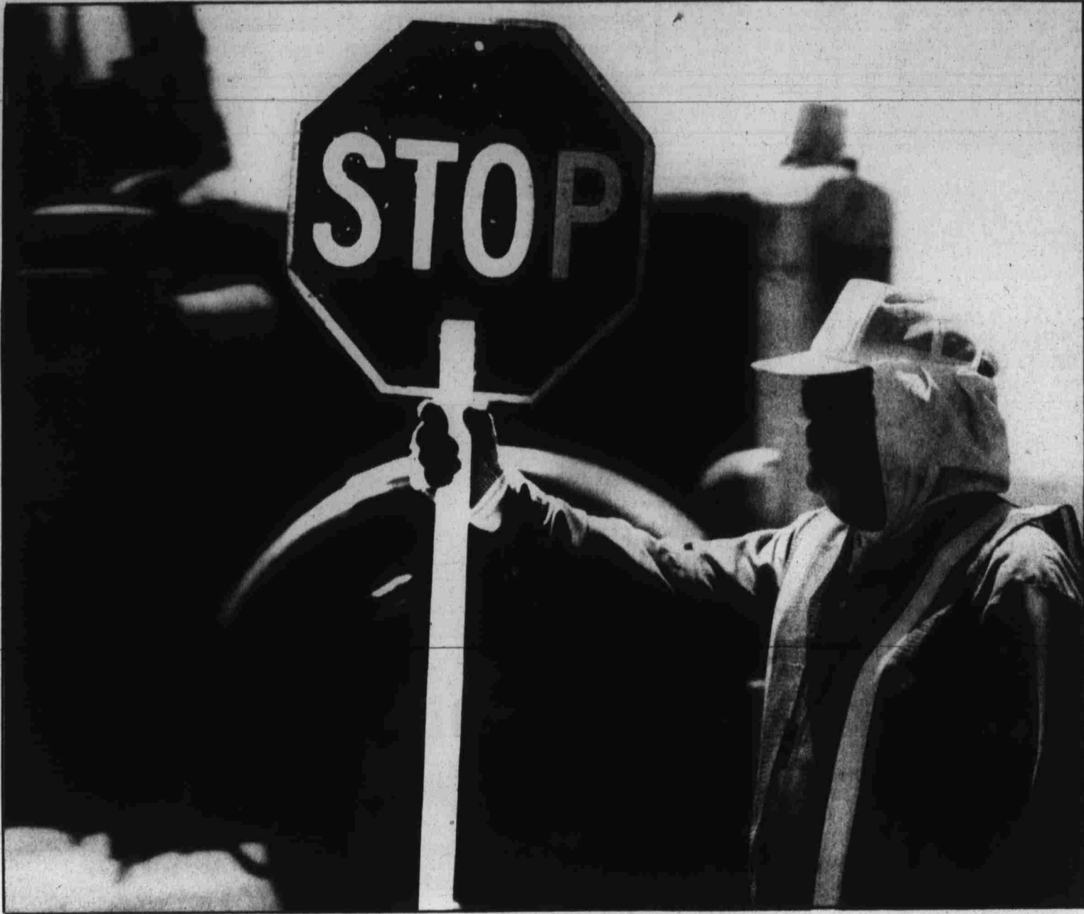
HOLD UP — Worker Ken Cooper shields himself from flying sand with heavy clothes Tuesday as he stops traffic on Stephanie Road while gravel trucks cross.
