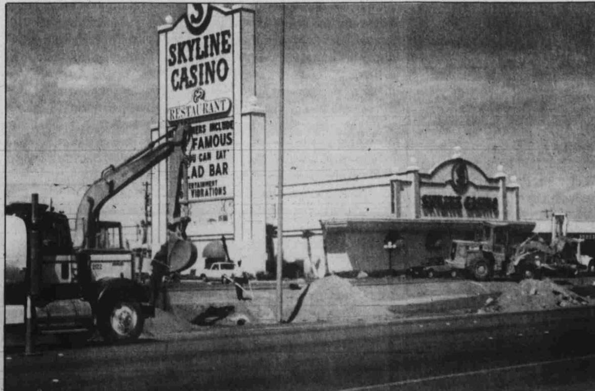
BEAUTIFICATION BEGINS —Construction trucks dig into the median islands of Boulder Highway in the Pittman neighborhood this week.
