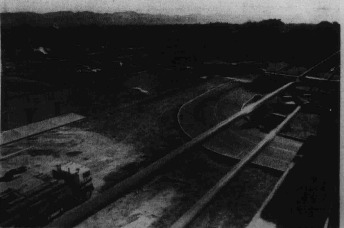
THE ROAD IN — The road into the parking garage is seen from the top of the building. Across Atlantic Street is the Henderson Convention Center, and Water
