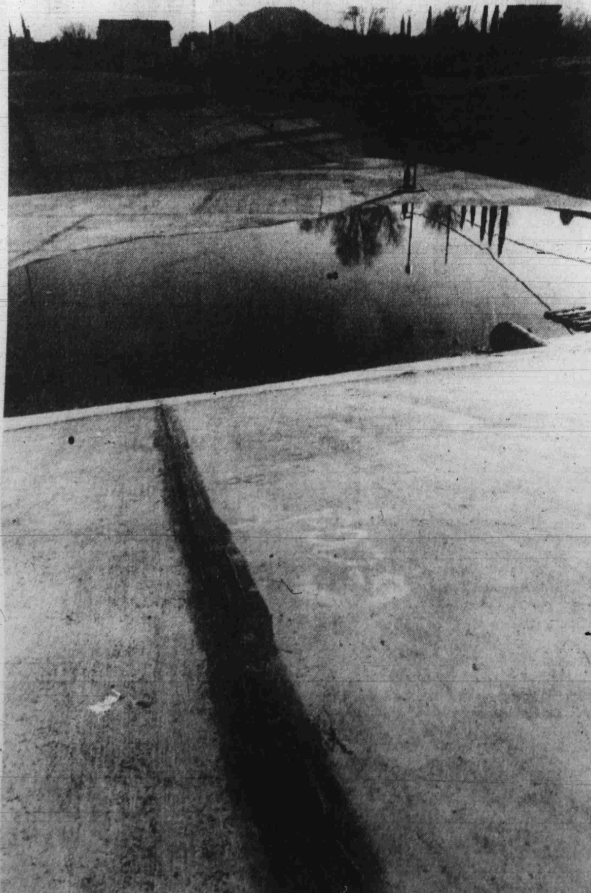
LEAKY SEALS —One of the two sealants used during construction of several reuse water ponds at Black Mountain Golf and Country Club deteriorated. The defective seams were repaired, and city officials report that treated effluent from the city's wastewater treatment plant began filling one of the ponds Wednesday. The treated water will be used to water the golf course.
