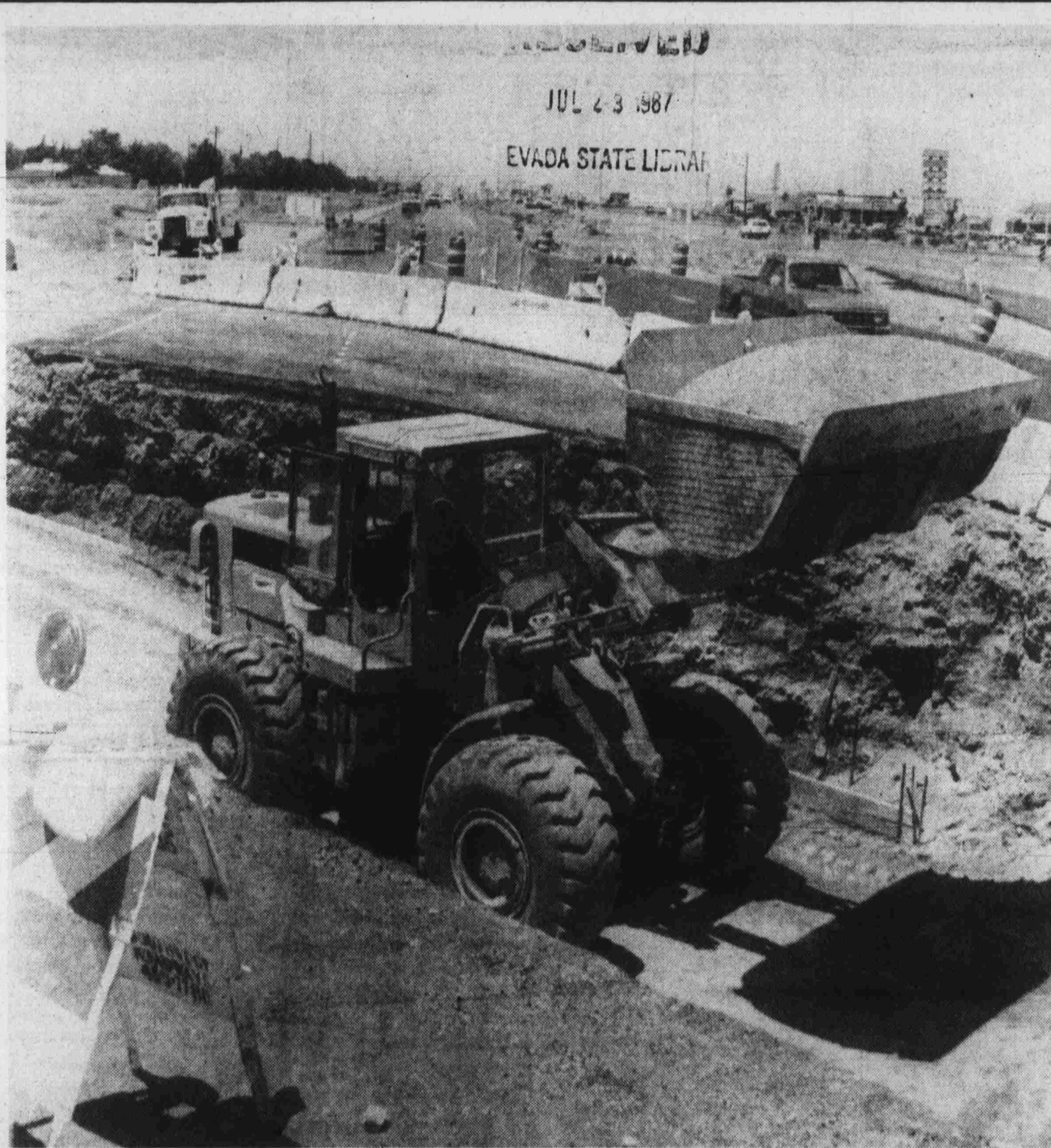
NEW FLOOD CHANNEL —Work on a new flood channel bound traffic near the Smith's Food King shopping center. Work is expected to continue for up to six weeks. Photo by Lee Quintance
