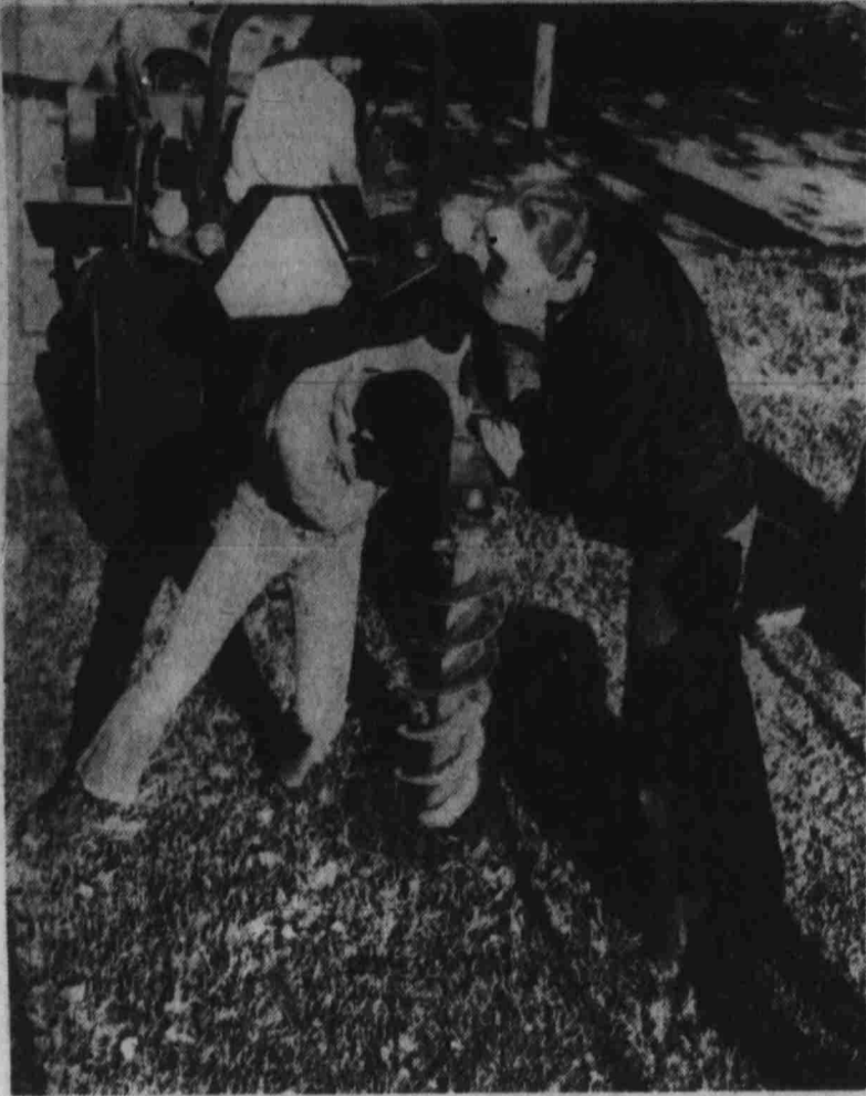
First the auger with assistants must dig holes for the equipment and signs...
