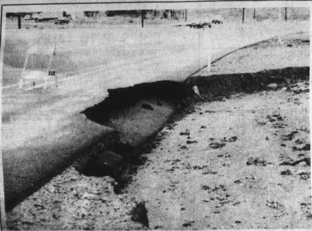
One of many pavement collapses on truck route
