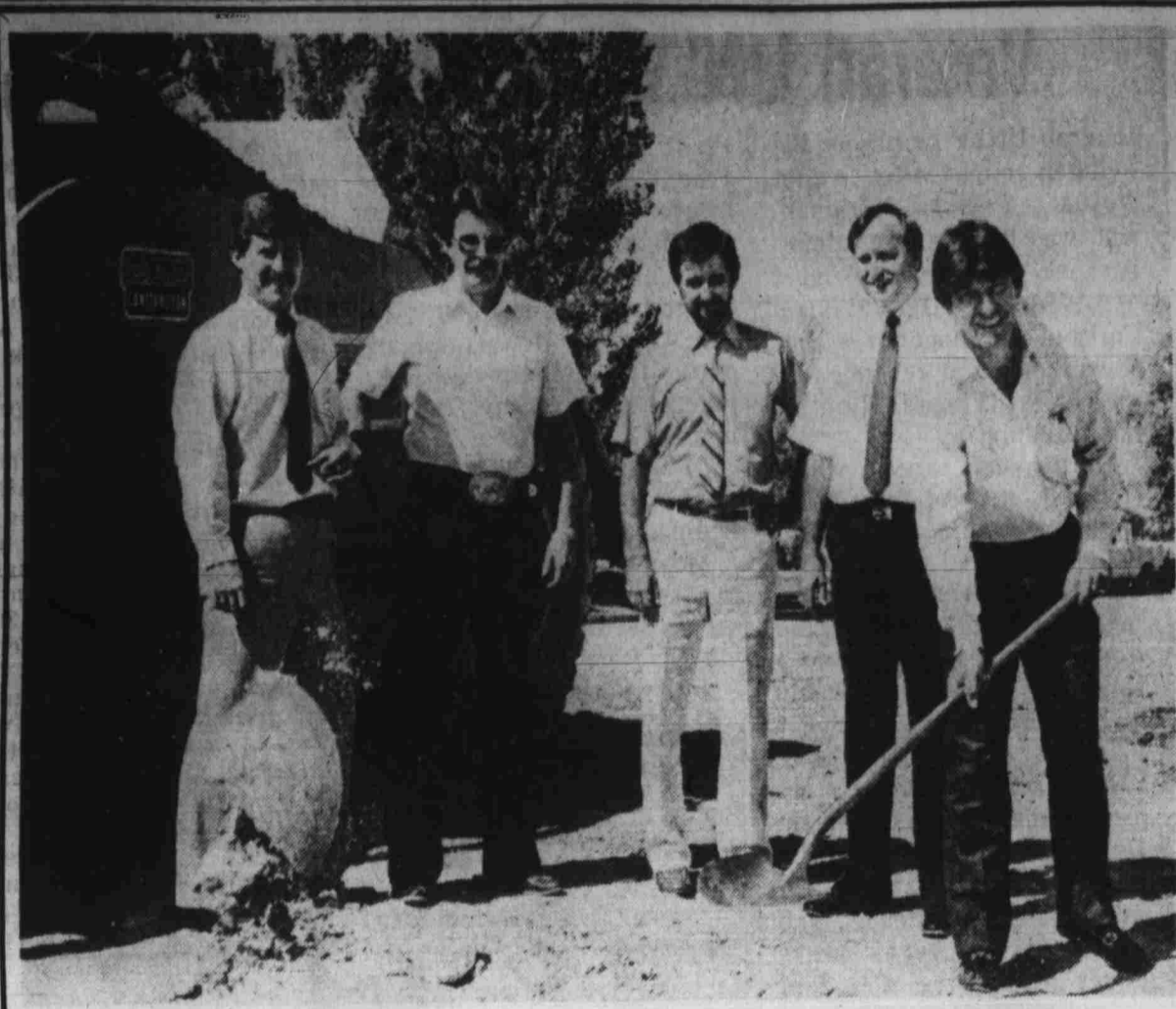
SHOVELFUL TO 13 YARDS - Architect Bob Kraft turns a shovelful of dirt for the first of three 10,000 square foot office buildings in Phase Two of the Green Valley Professional Center. When completed, the entire complex will cover 55,000 square feet and will be the largest office facility in Southern Nevada, south of Tropicana Avenue. Also pictured, from left to right, are Brad Nelson, vice president of planning for American Nevada Corp., Frank Martin, Martin-Harris Construction; Mike Koizume, VTN Engineering and Bob Campbell, senior vice president, American Nevada Corp.
