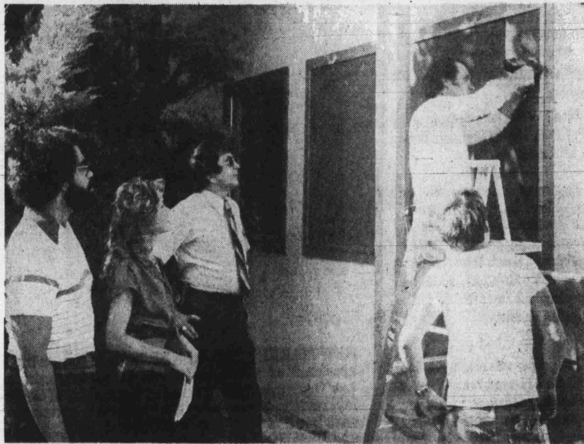
SOLAR SCREENS INSTALLED -- Solarex, Inc., is shown installing solar window screens at city hall. Left to right are Jim Gardner, Linda Mann and Julius Conner. On the ladder is Chuck Fox and standing is Keith Yoder.
