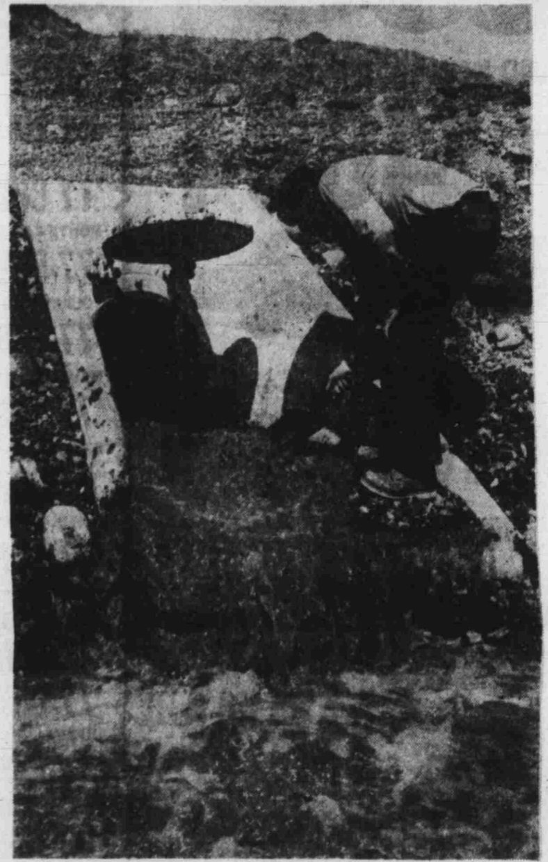
RUSS COGGINS cleans debris away from the end of the drain pipe as water rushes forth. The increased flow is due to the gate being raised for scraping.
