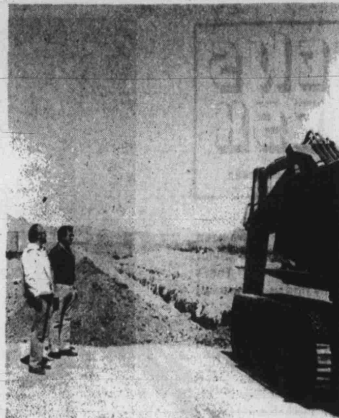
TRENCHING STARTED - A trench is being dug along Greenway Road for an 18 inch Water line which will provide water for the lower part of the Paradise Hills subdivision, Mission Hills and the industrial area which includes Levi Strauss. Joe Bachman and Ross Howes of the Paradise Hills sales office observe as work progresses on the much needed line.
