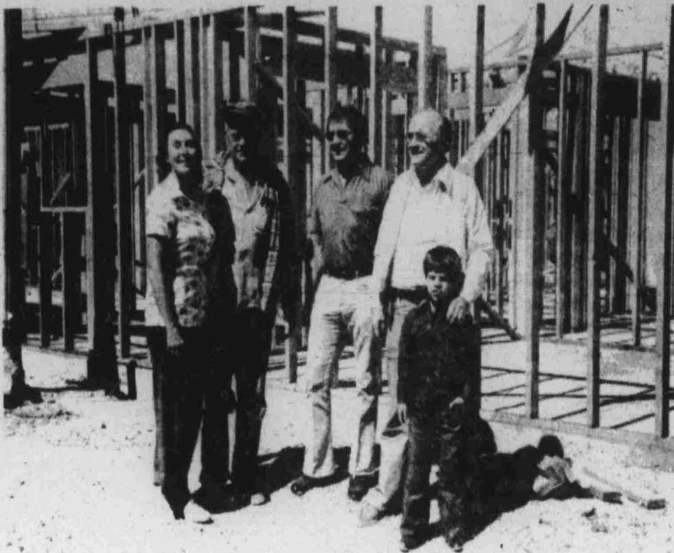
NO ONE COULD BE PROUDER - Elois and William "Bill" Barton, left, stand happily in front of their new home which is now under construction in Paradise Hills. With them are Ross Howes, Fidelity Realty Co. Sales Counselor, Jess Bachman, Project Manager for Paradise Hills and his grandson.
