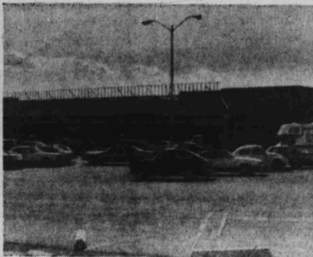
MORE RENOVATION - The addition and renovation to the Safeway Store on Nevada Highway is progressing smoothly. The enlarged store will also sport a new front as shown above.
