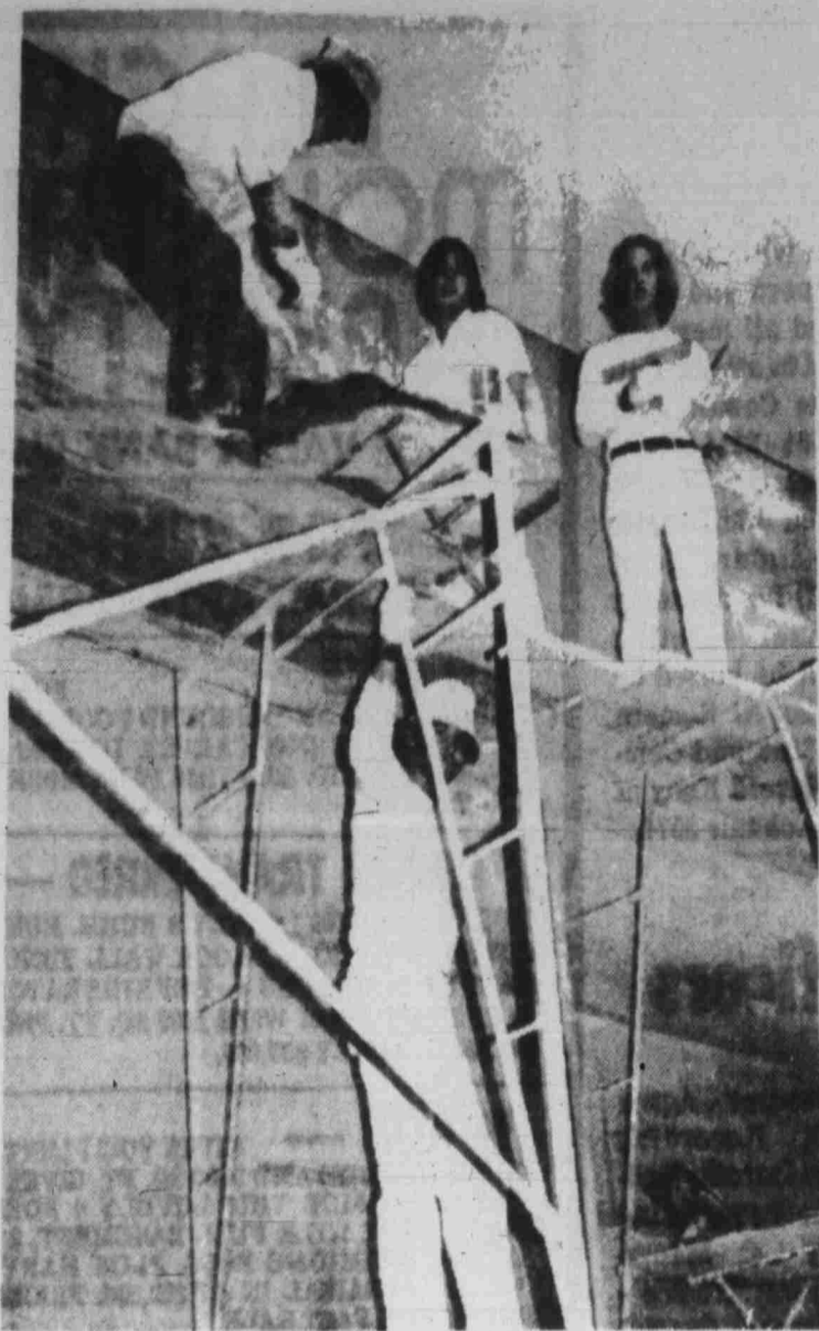
BOYS' CLUB HANDBALL COURT GETS PLASTERED - Fifteen senior apprentice plasterers from Local No. 797 have been working very diligently the past three days applying plaster to the walls of the new handball court which is nearing completion at the Boys' Club. Two instructors and the business manager and business agent for the Plasterers and Cement Masons local have been overseeing the job which has been of great benefit to the Club.
