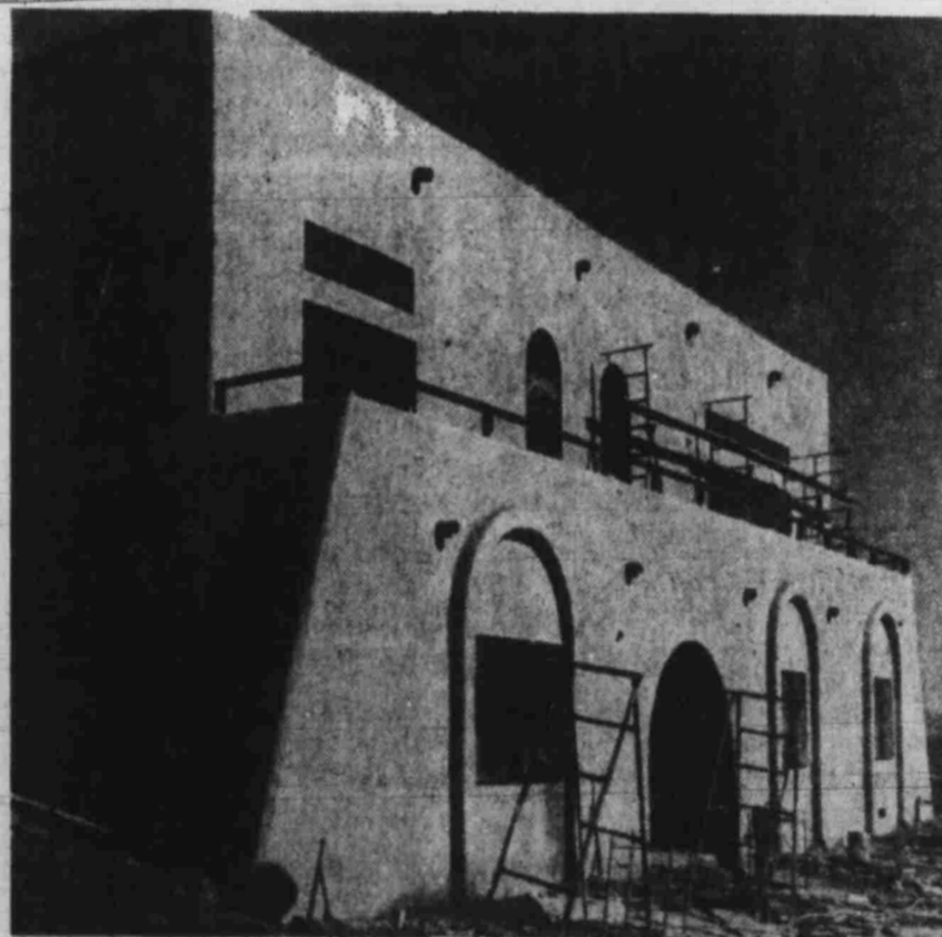
PORCH WITH A VIEW - This custom built home on Keys Drive in the lower portion of Hemenway Valley has a mountain back drop and an open view of Lake Mead. It is but one of several homes now under construction.
