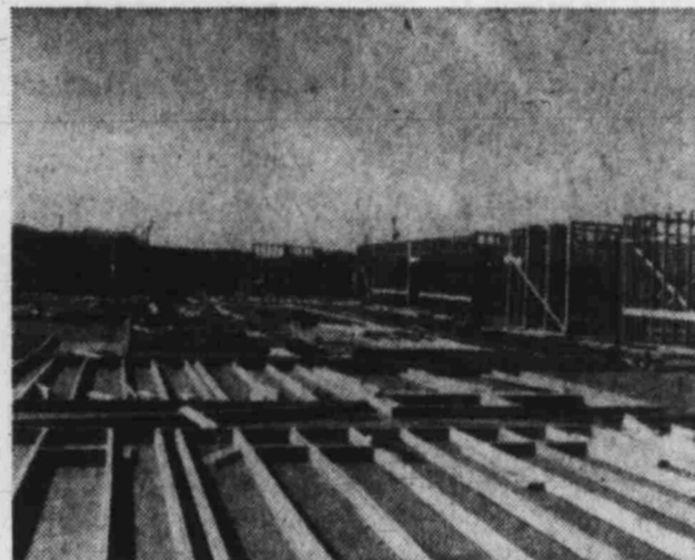
LOTS OF LUMBER - The convalescent home designed by Careage Corp. at the corner of Adams and San Felipe is now at the stage of construction shown above with walls springing into place.
