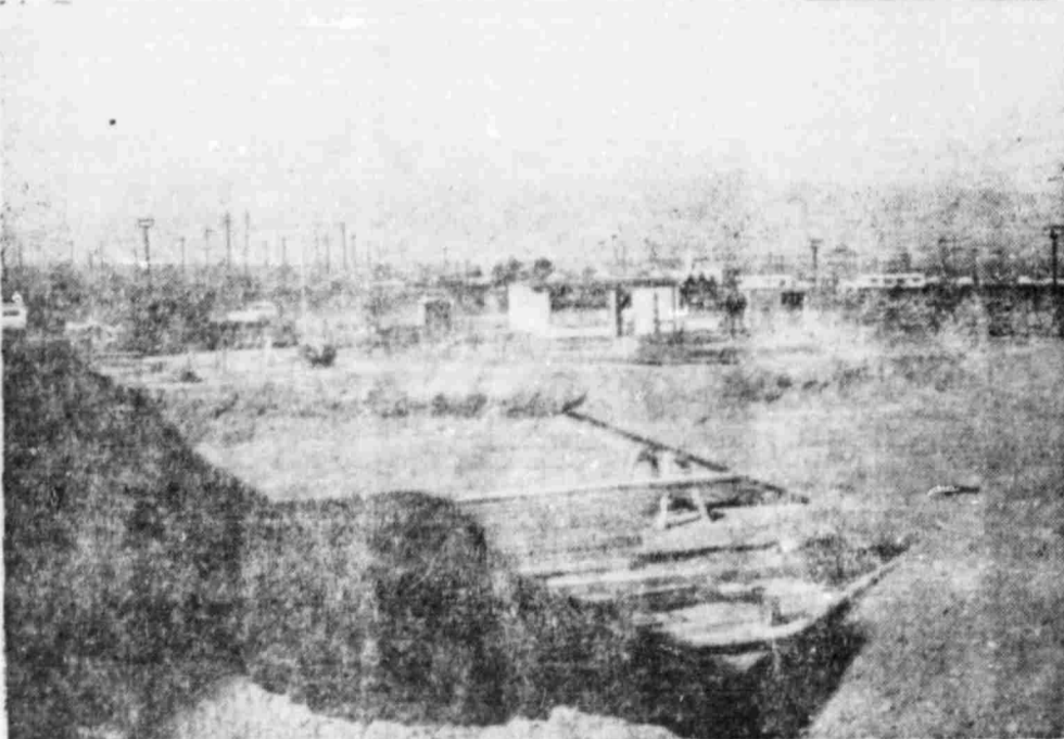
A 'HOLE' LOT OF ACTIVITY -- Work is well underway on the new swimming pool to be located adjacent to the gymnasium at Basic High School. The pit which will contain the pool itself has been dug and the foundation footings of the building which will encase the new aluminum pool have been poured, giving a viewer an idea of the size of the structure. According to authorities, work is going along on schedule.
