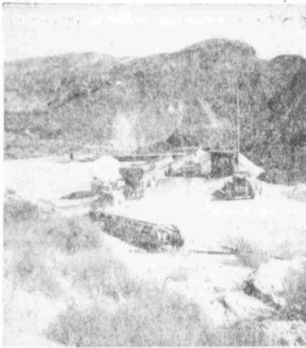
HENDERSON BREAKTHROUGH —A revolutionary new concept of on-site ore extraction known as the Spendlove Dual-Reduction Process was developed and begun by a group of local people here in Henderson. The site above shows a larger "mill" in operation in Hurricane, Utah.
