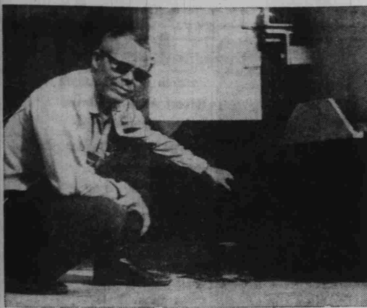
Mechanical engineer James N. Peterson is shown on the transformer deck at Hoover Powerplant. His hand resting on one of the transformer rail stops. Modification of these rail stops, to decrease the possibility of movement in the event of a severe earthquake, has been the object of a recent study. Jim, whose job is solving problems such as these, was recently presented a 10-year length-of-service pin.
