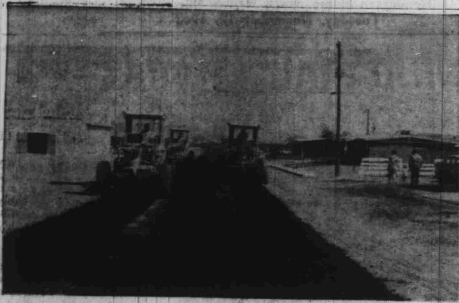
MIXING BOWL —Four road graders are shown mixing the blacktop on Corn Street. The oil and gravel is turned over and over then left in a row down the center of the street to soak for remixing.
