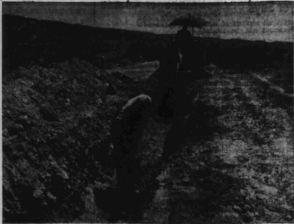
THE TAIL END —The ditches for the mains to supply water for Industrial Park Development Project, south of Sunset Street and west of Boulder Highway. The water mains, 12 inches in diameter, have been laid a mile and a half into Industrial Park, up to Gibson Road. HOME NEWSphoto
