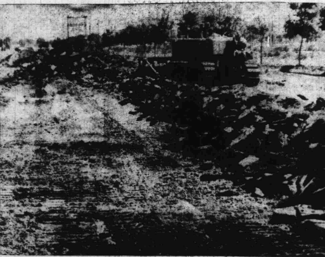
RIPPING UP BLACKTOP — Heavy equipment is shown ripping up the blacktop on the Water Street extension preparatory to improving the street. The county is doing the work for the city under a prior agreement.
