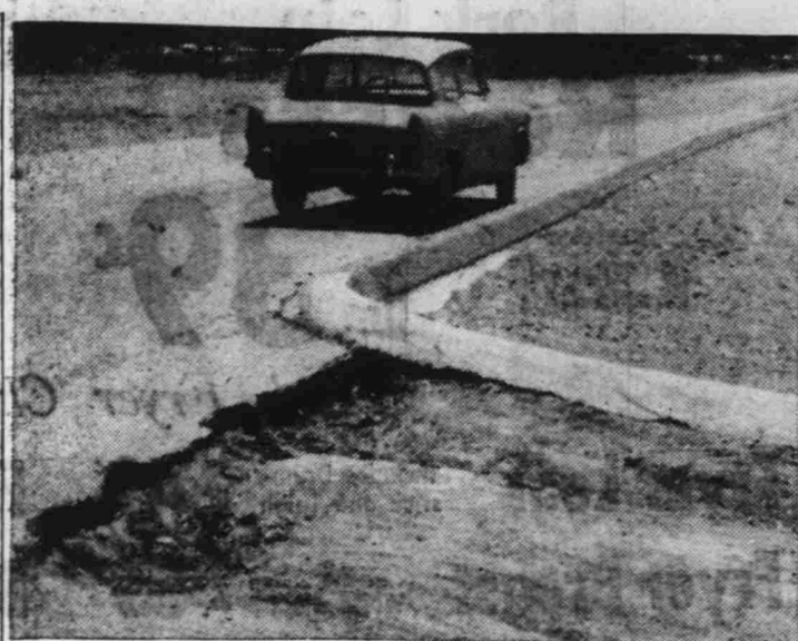
TIRE BUSTER — Who maintains the access roads? asked our advertising representative after encountering this chuck hole on the approach to the access road between Victory Village and Vegas Wash Road in the vicinity of Trailer Haven. After looking at the picture she took when she stopped to check her tires—we could only answer — "from the looks of this, no one."
