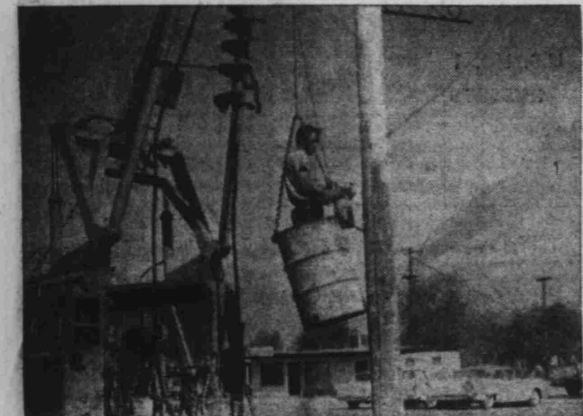
WHEN THE LOCAL CAL-PACIFIC power company started to re-paint some of its power poles this week, a NEWS photog happened along and shot the quaint way the company arranged for the painter to relax and enjoy his job in comparative safety. As shown above, the man just stands in a barrel—and what could be safer?
