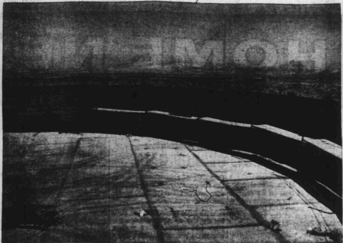
HERE IS THE INSIDE STORY of the new water reservoir now being constructed behind the golf course to supply better water pressure and more homes with city water. The reservoir will be 40 feet high—what you see here is the tank after its first eight foot sheet has been installed. It'll take five high of these plus a roof before it will be ready to hold a million and a half gallons in storage.
