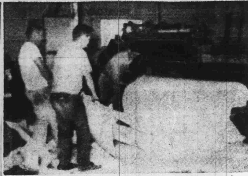
Workmen are shown adjusting parts, now in place on the new HOME NEWS press. Everything must be perfect, if the machine is to work properly. Home News Photo
