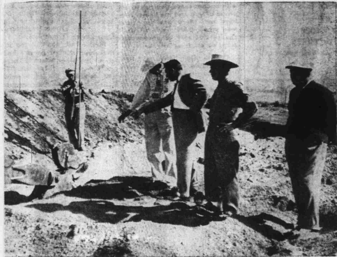
SEWER WORK STARTS — City officials and Pittman property owners met Tuesday at 9 a.m. in Pittman for ground breaking, as work on the sewer lines was started by George E. Miller Construction Company. Shown above, left to right, are a Miller Construction employee, measuring the depth of the ditch being dug by the big back hoe; Robert Cordill, City Engineer and Ward Five Councilman Lou F. La Porta, who can be seen checking the water table; Councilman Aubrey Pagan and Gene Ward, Pittman's largest property owner. Also present were Mayor Bill Byrne, Councilman Robert Kesterson and Robert Pfluger, owner of the Swanky Club. Gene Ward attended the first ground breaking in this area 30 years ago. He recalls that Moser and Bearden, the first subdividers in this area—then known as Jericho Heights — had a band and great festivities as they started the sub-division, now called Midway City, with lots selling for $400 each.
